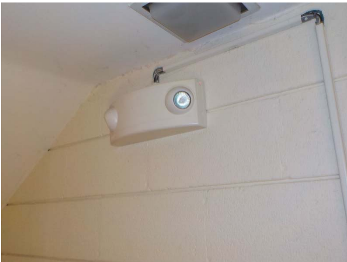
View of emergency light at Church basement stairs.
