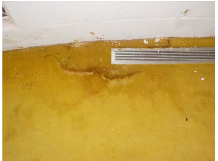
View dated carpet with water damage in the Church.
