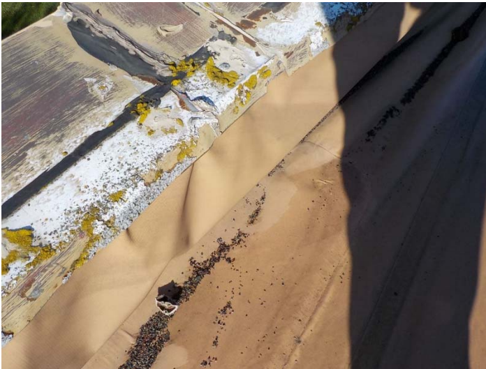
View of damaged roof flashing.
