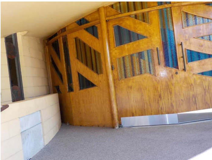
View of Church entrance doors, requires refinishing.
