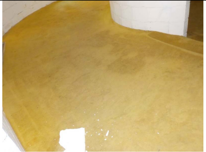
View dated carpet with water damage in Church.
