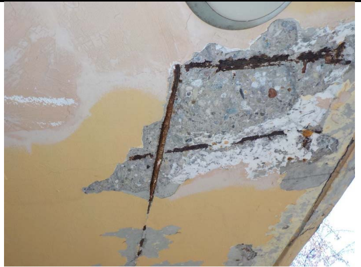
View of delaminating concrete at Church entrance.
