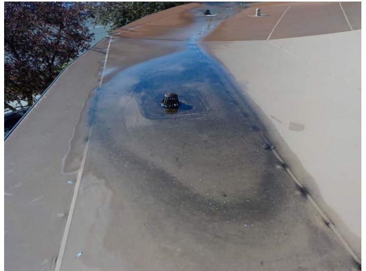
View of ponding at roof drain.
