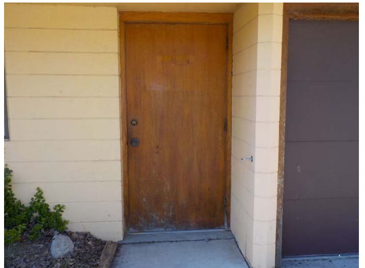
View of entrance doors, requires refinishing.
