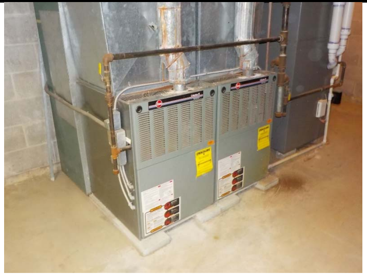
View of forced hot air furnaces for Rectory.
