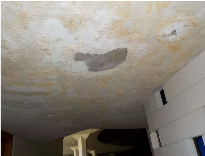
View of damaged plaster in Church.
