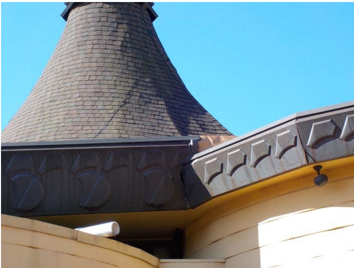
View of ageing (degraded) Church steeple.
