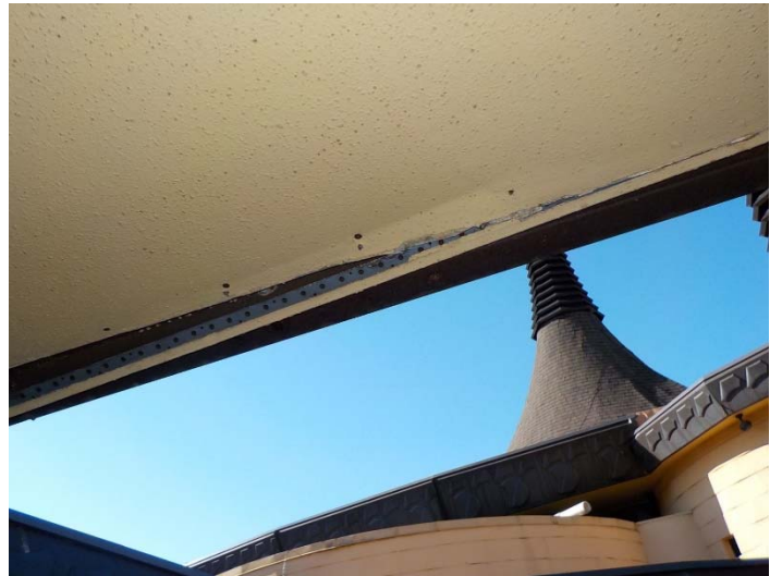
View of damaged soffit at Rectory.
