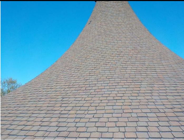
View of steeple roof with missing shingle.
