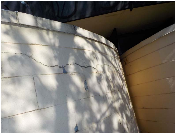
View of damaged block wall at the Church with stress crack.
