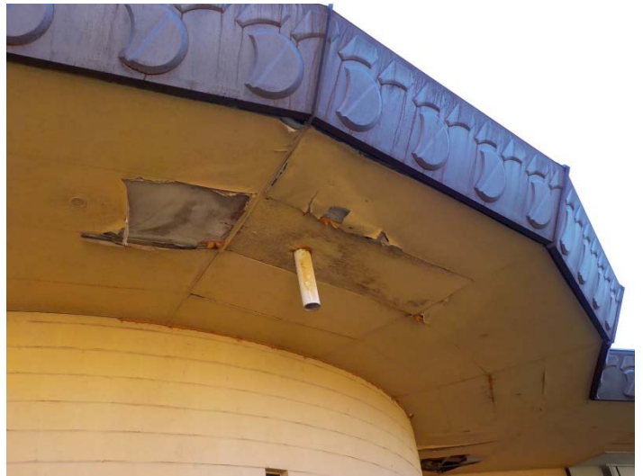
View of damaged soffit and inadequate roof drain.
