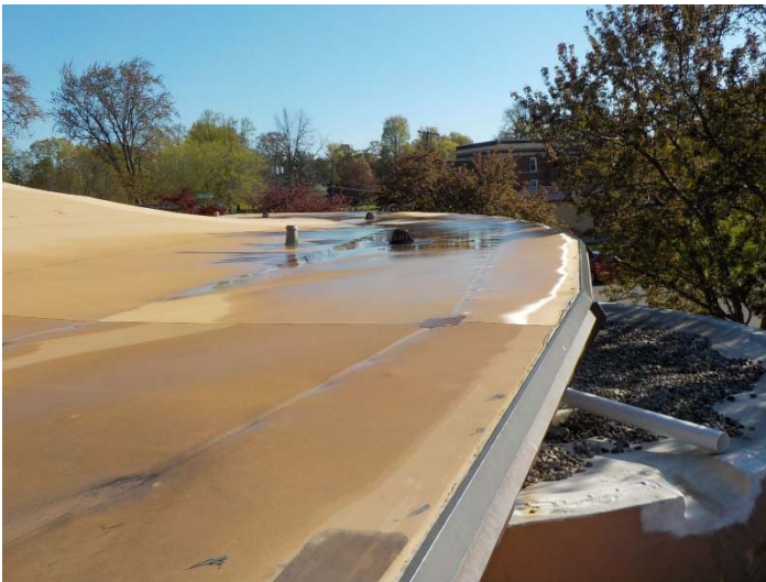
View of membrane roof with ponding.
