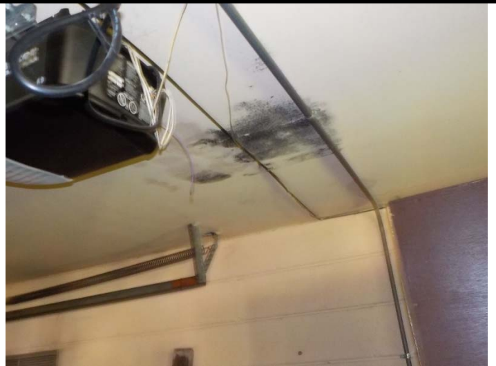
View of mold in the Rectory garage.
