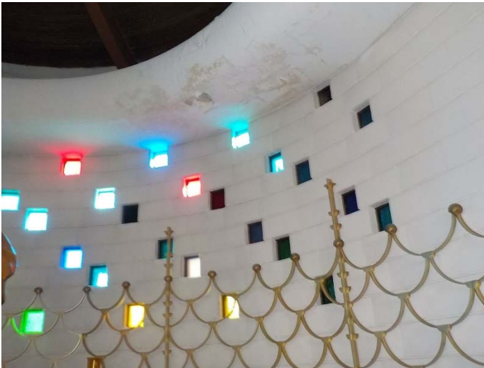
View of water damaged ceiling plaster in the Church.
