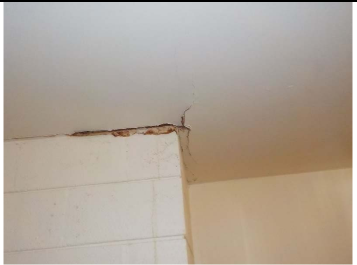
View of roof leak in Rectory.
