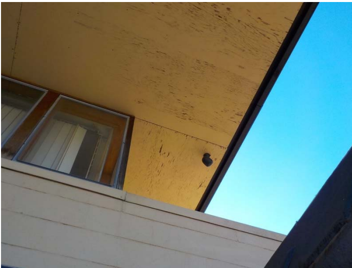
View of soffits requiring paint at Rectory.
