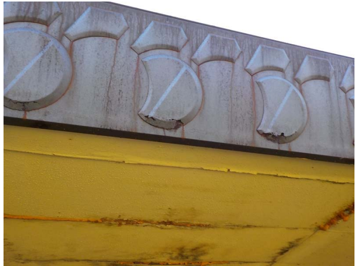
View of oxidized (rusting) fascia and damaged soffit at Church.
