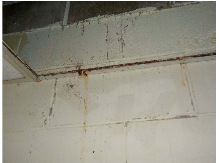
View of water infiltration area in Rectory basement.
