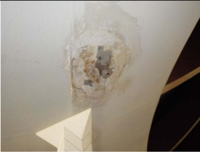
View of damaged plaster in the Church.
