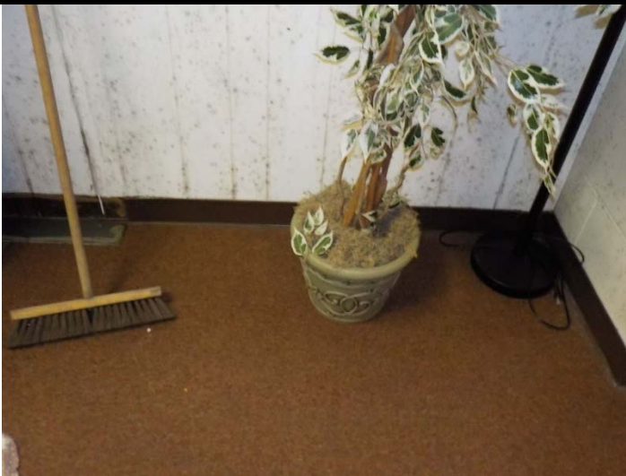
View of mold in the Rectory basement.
