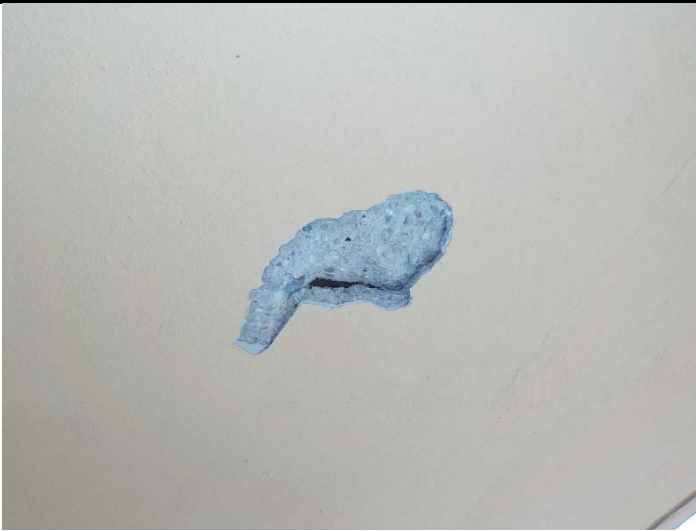
View of delaminating concrete at Church entrance.
