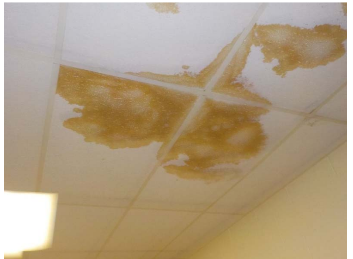
View of water damaged ceiling tile in Rectory basement.
