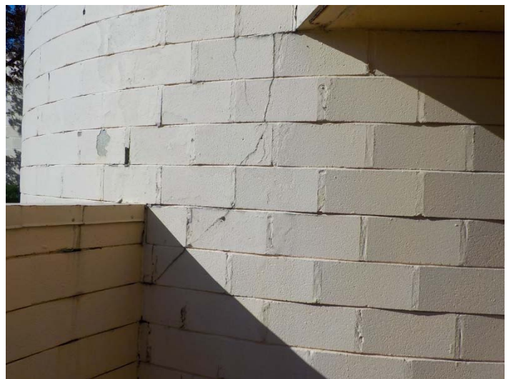
View of damaged block Church wall with stress crack.
