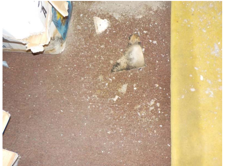
View of failing plaster in Church.
