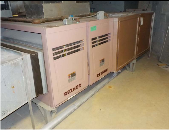
View of boilers for Church.
